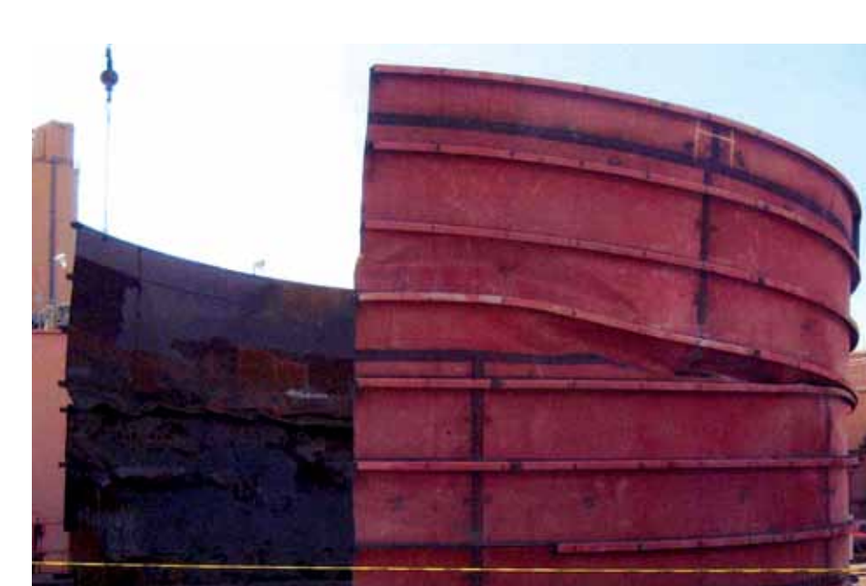
Significant material loss can cause the chamber to fail.
