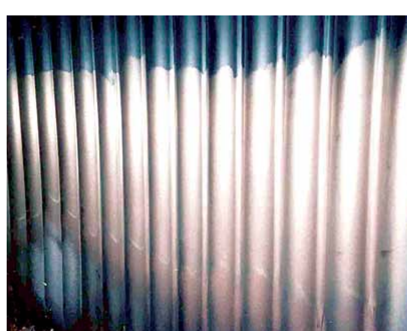
NanoSteel SHS 7170 TWAS coating shows no erosion or corrosion damage.
