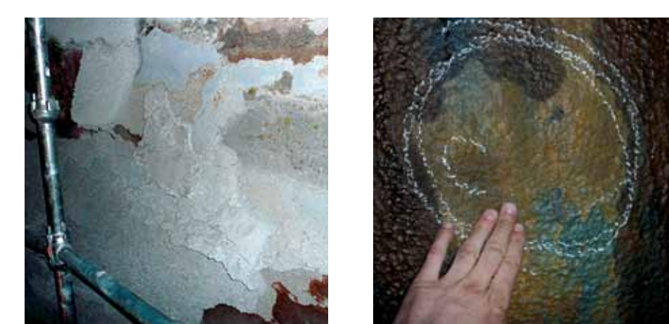
Corrosion scale, fly ash and lime milk build up on chamber ID wall.
