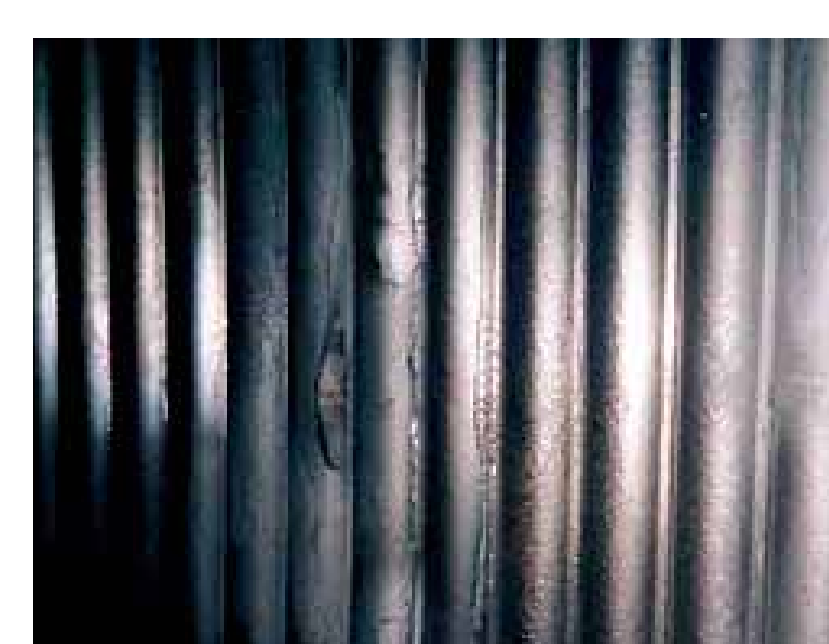
Competing steel coating shows damage from erosion requiring repair.
